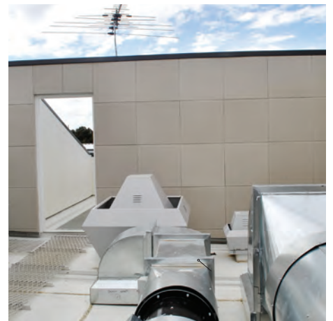
Cooling towers and HVAC
