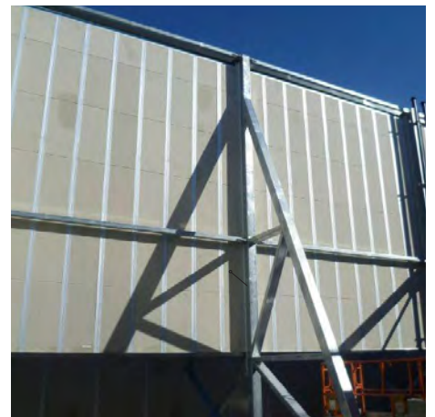
Outdoor areas - including Power generators, air conditioning enclosures
